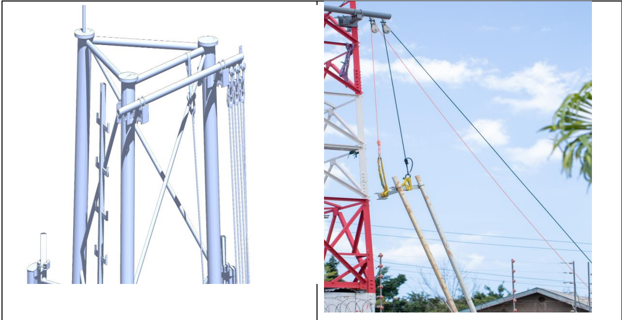
Figure 8.2 & 8.3 The Gin Pole or Derrick (Lifting Beam) is to be set up on the top of the tower to accommodate heavier loads to be lifted. The Gin pole must be installed and secured across the two tower legs and be fitted at the end of it with an eyelet, shackle and pulley for the pulling rope.
