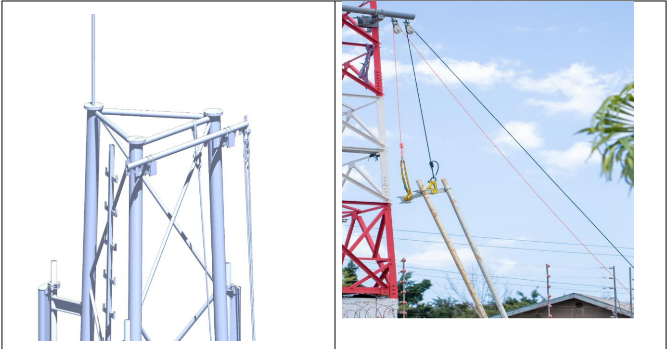
Figure 7.2 & 7.3 Gin Pole or Derrick (Lifting Beam) must be set up on the top of the tower to accommodate the heavier loads to be lifted. The Gin pole must be installed and secured across the two tower legs and be fitted at the end of it with an eyelet, shackle, and pulley for the pulling rope.
